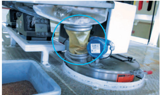
VIBRATORY SCREEN DISCHARGE TO AUGER FEEDER INLET - AFTER
