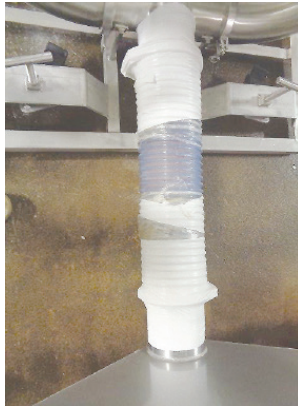
Original connectors were often taped to prevent leakage
